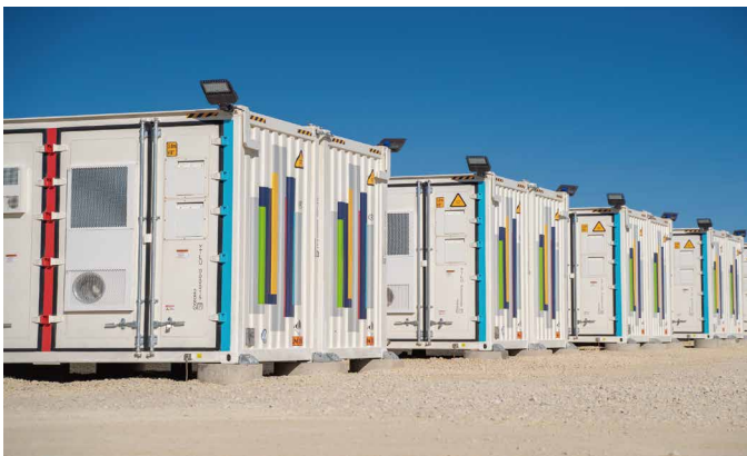
Texas, USA 226MWh Frequency Regulation
